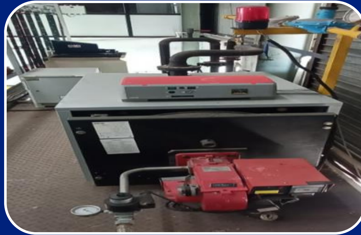
Hot Water Generator
